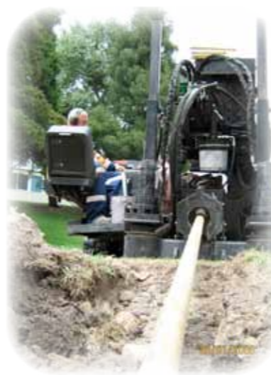
▲ Ditchwitch 30/20 drill rig utilised to drill down to and intercept the existing pilot hole
