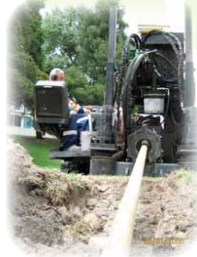
◀ Ditchwitch 30/20 drill rig utilised to drill down to and intercept the existing pilot hole
