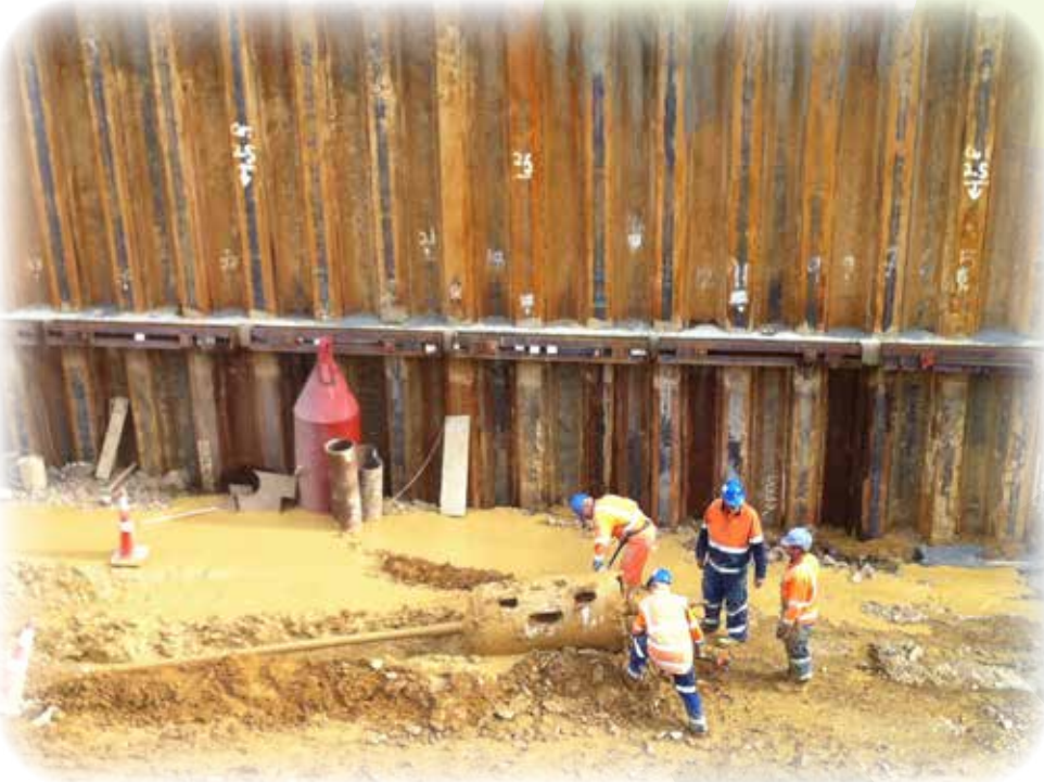
▲ Barrel reamer utilised to counter sinkage in the soft ground sections of the 200m long drill shot
