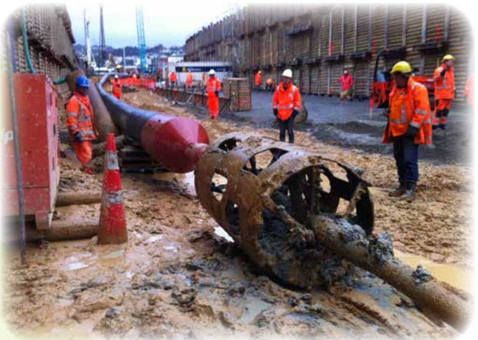
▲ The 710mm diameter polyethylene pipe is connected to the barrel reamer and drill string ready for installation
