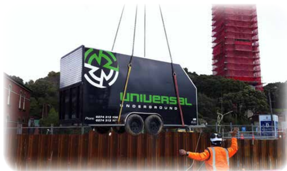
▲ Access was difficult- It was necessary to crane support equipment into the trench.
